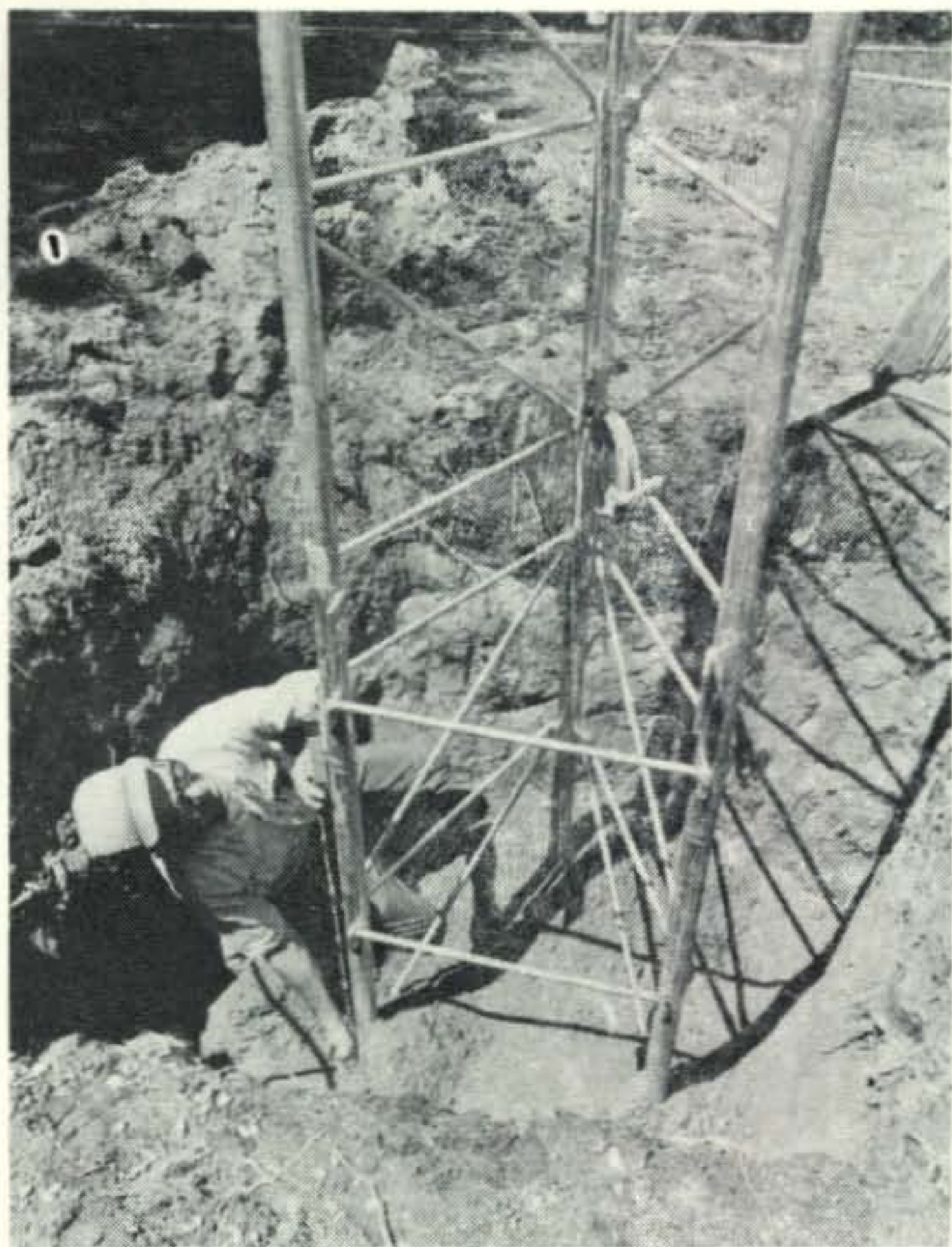
The base is set in the hole and positioned properly with respect to the edges. It is not set dead center (see text and fig. 1). Check orientation also to be sure of clearance for tilting. Tower tilts toward the point of the open vee.
