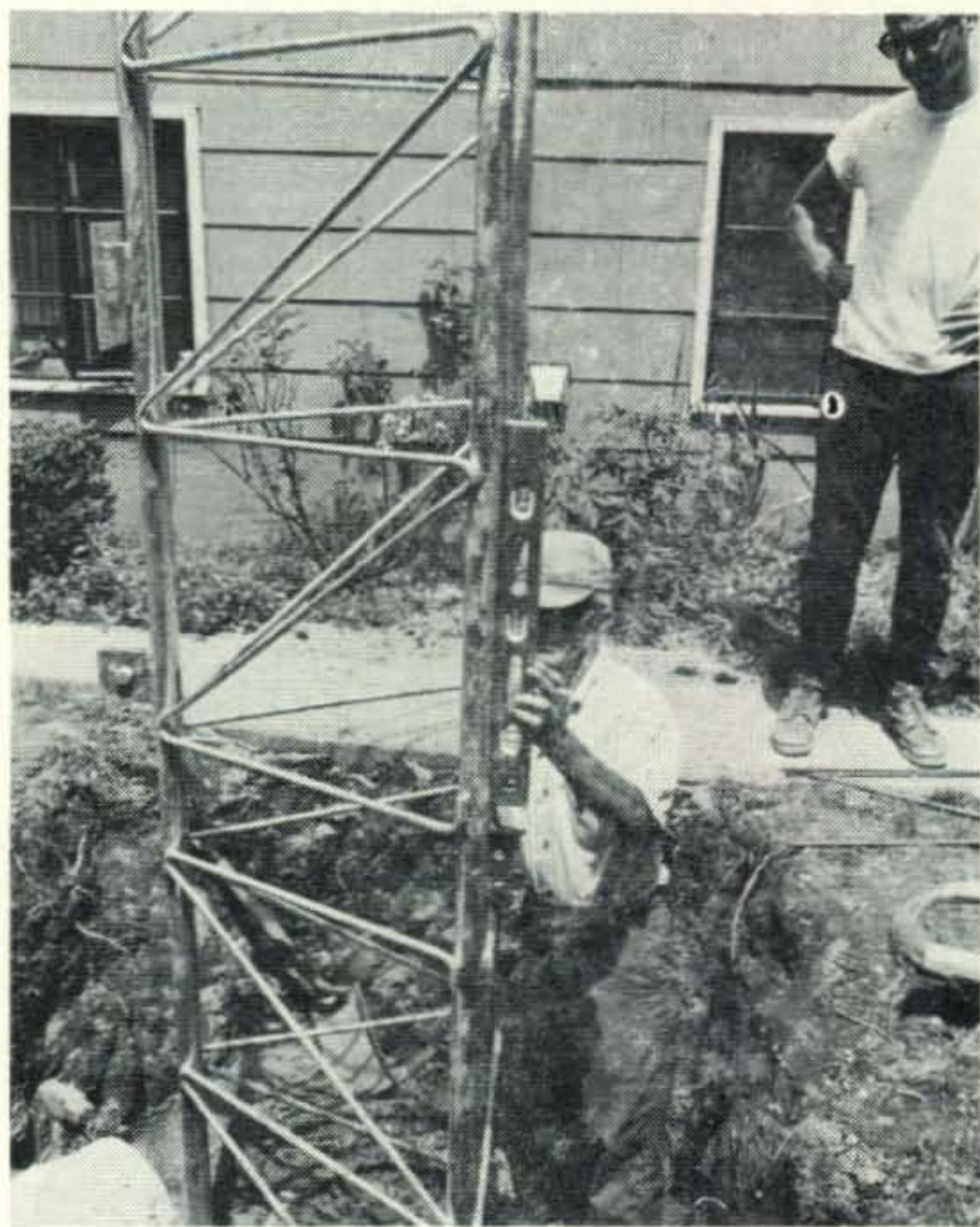
Drainage for the pipe legs must be provided to prevent water from accumulating inside and rusting the pipes. Fortunately, the bottom of this hole was pure sand and nothing else had to be done. The base is seen here being leveled before the concrete arrives.
