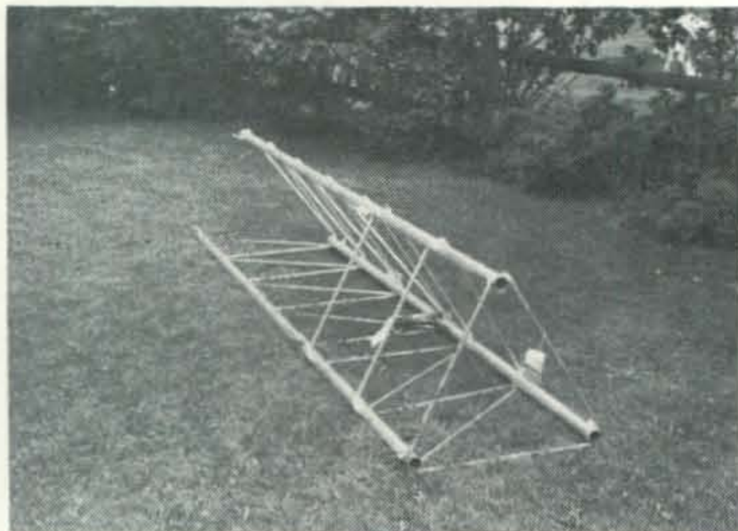
Massive base is constructed of heavy steel galvanized pipe and solid rod braces welded to uprights. Enclosed area in foreground goes into the concrete. The open vee protrudes above ground and enfolds the tower.
